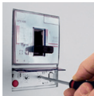
< Adjusting the magnetic threshold of a DPX circuit breaker
