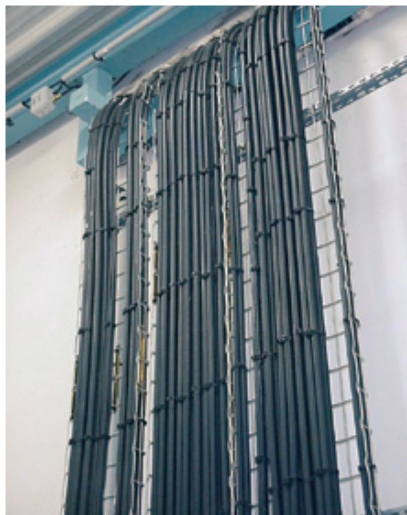
^ A neat cable layout is essential with regard to the fire risk
